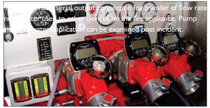
East Sussex Fire and Rescue Service Year 2007 fire appliance pump bay.
