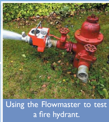
Measuring static and dynamic pressure and flow rate.
